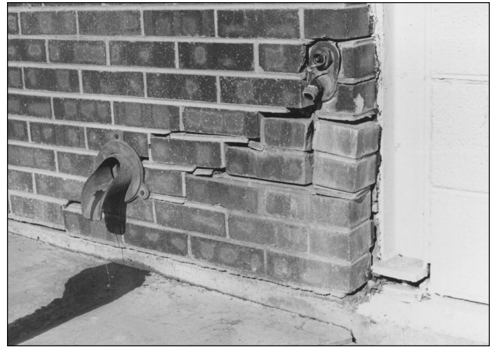
Damage to foundation and mortared brick walls from settlement of collapsible soils. Building in Montrose was demolished shortly after photo was taken. PHOTO COURTESY OF BUCKHORN GEOTECH
