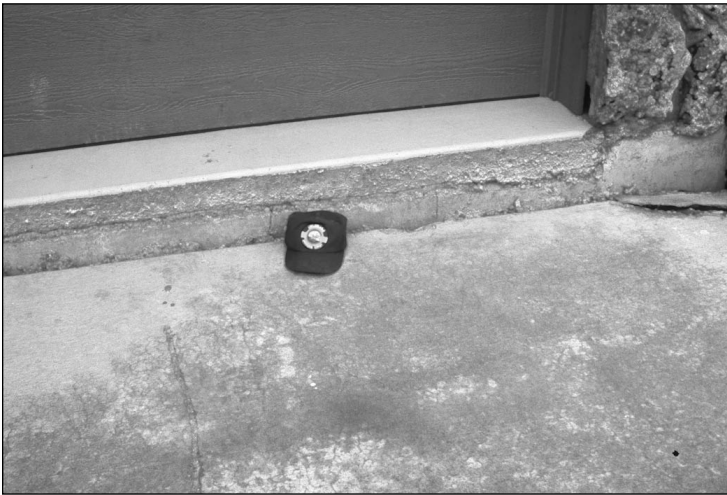
Continued settlement in collapsible soil dropped new town-home driveway to a level where vehicles are unable to enter garage. Note leveling slab of concrete on garage floor from previous repair.
